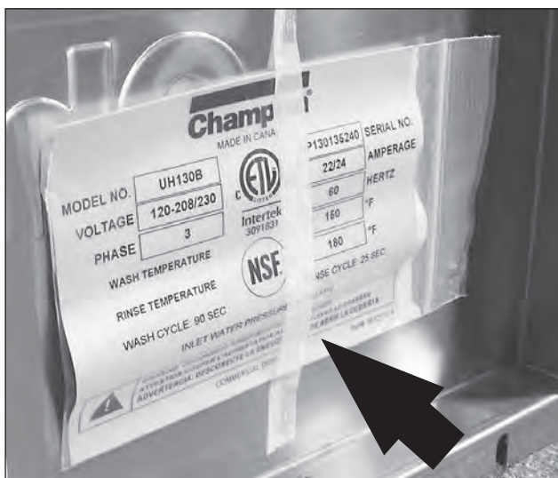
A replacement three phase data plate is stowed on the back of the machine lower front access panel.
