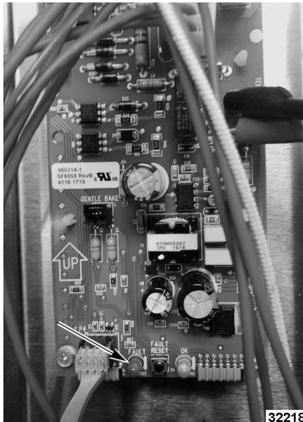
LED FAULT INDICATOR LIGHT ON BOARD
